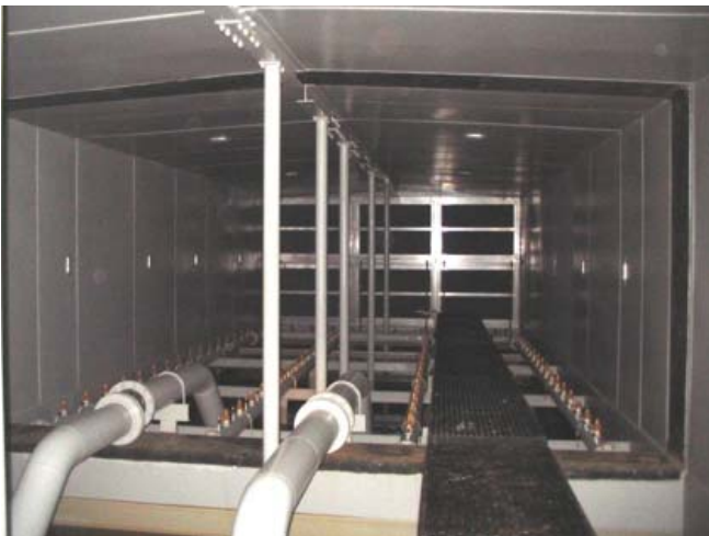
FIG 15 - Photograph of north air cooler.
