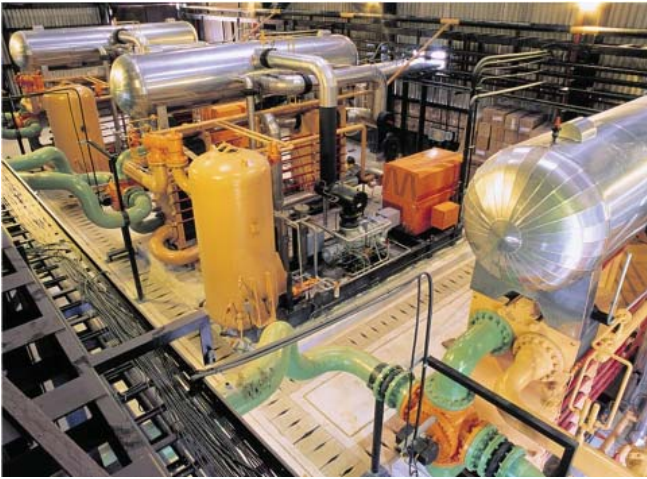
FIG 8 - Refrigeration machines (NH 3 ) for first phase.
