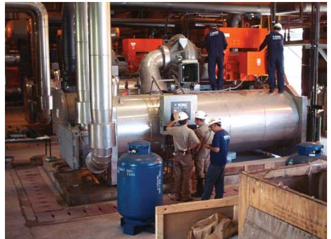
FIG 9 - Refrigeration machines (R134a) for second phase.
