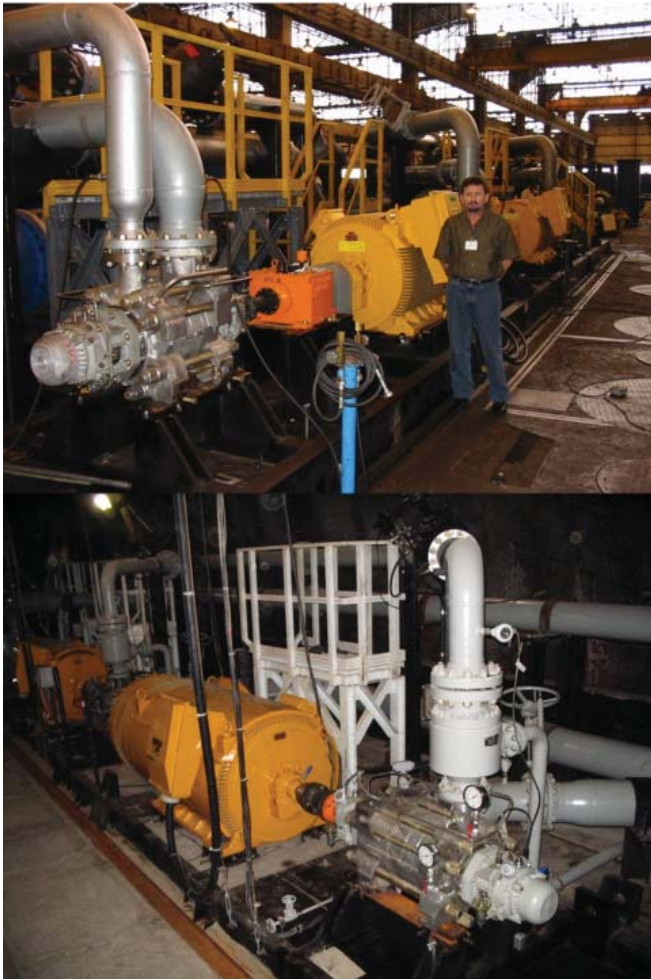
FIG 17 - Energy recovery turbine and return pump.
