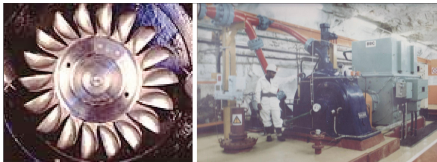
Figure 11. Typical turbine generator systems (5 MW rating)
